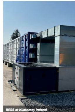
BESS at Kilathmoy Ireland
