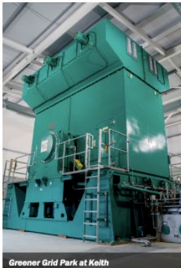
Greener Grid Park at Kelth
