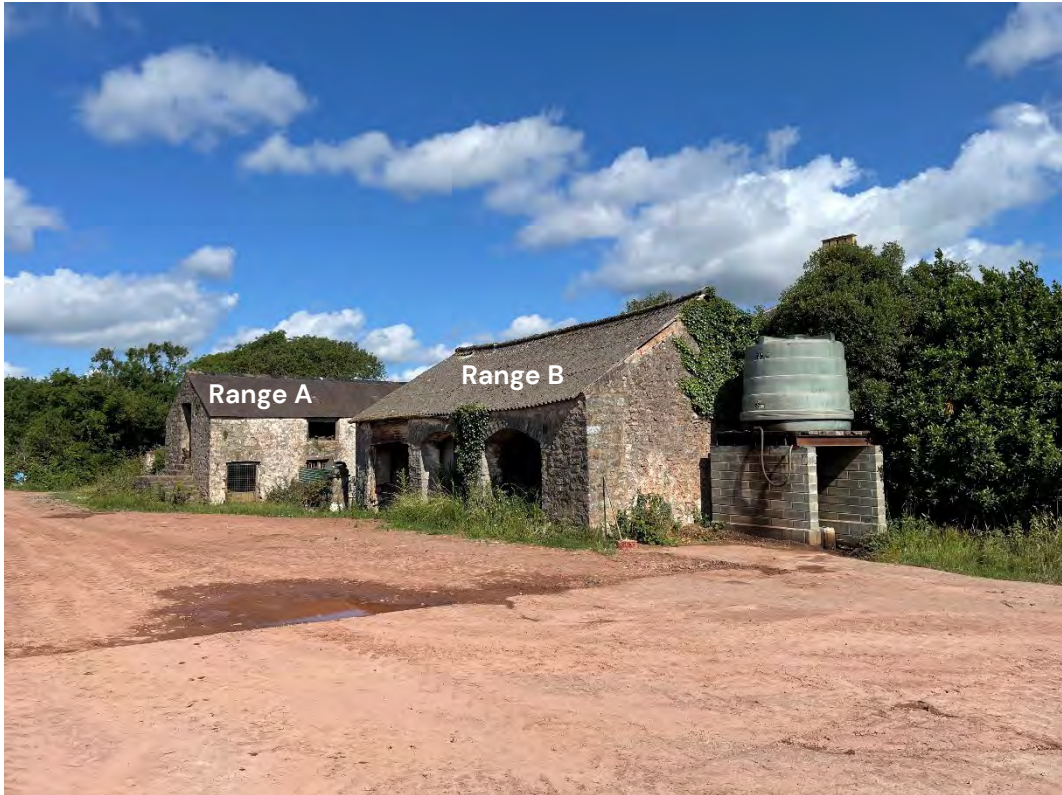
Plate 1: Historic outbuildings to the rear (south) of Alleston Farmhouse, looking north-west from where the farm access track enters the farmyard
