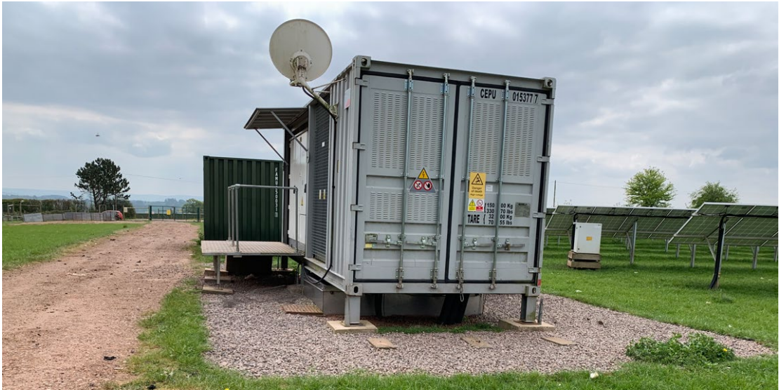
Inserts 22: Typical Inverter Container (example from Monmouthshire)
