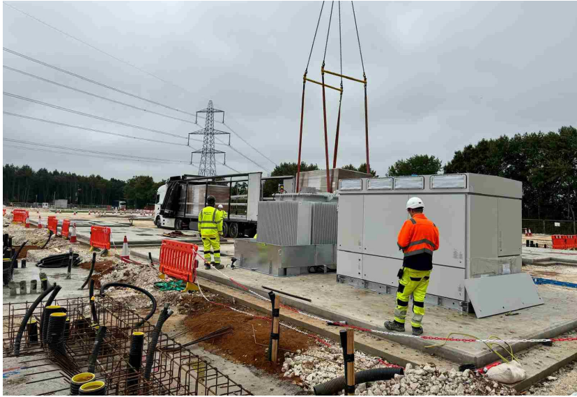
Power Conversion System Delivery 26/09/2024
