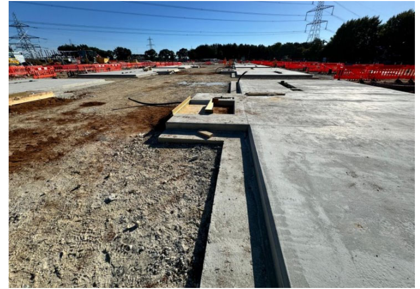
Cast Ring Main Unit Base Extension 19/09/2024
