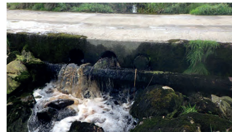
Figure 35: Poorly designed road bridge
