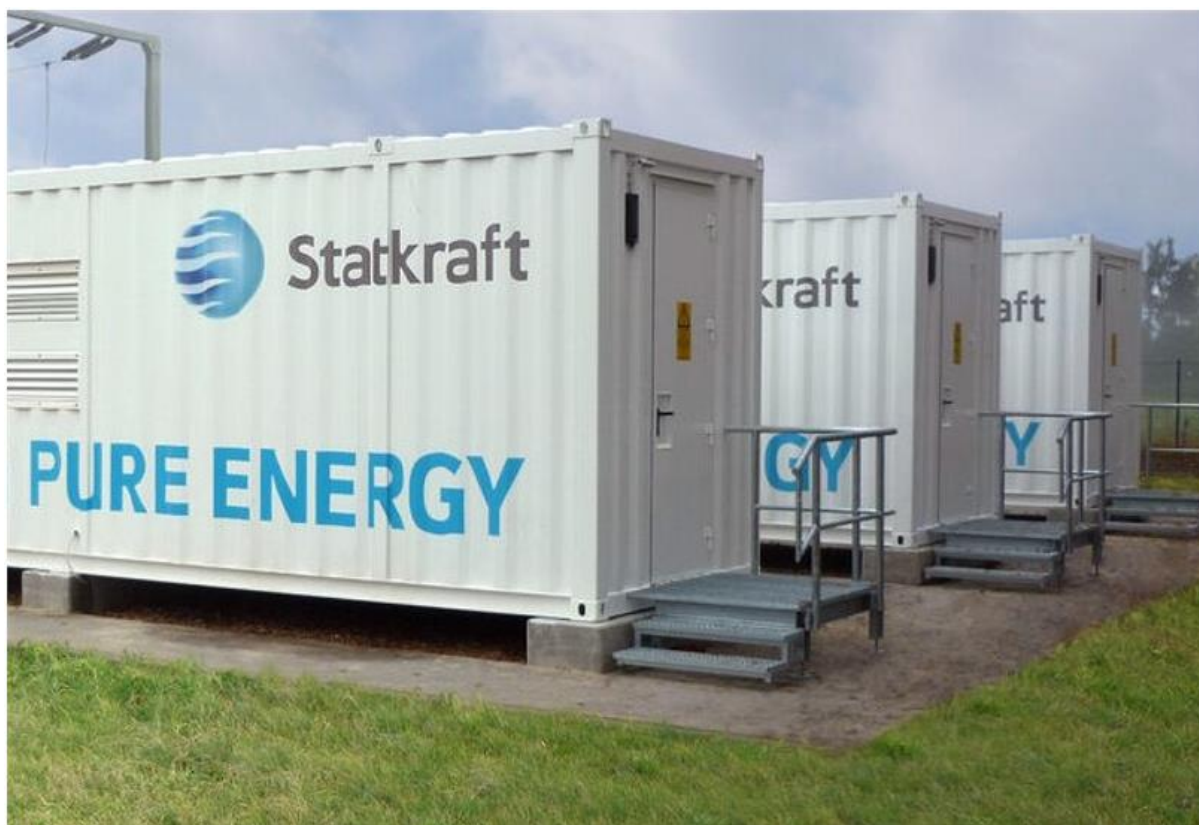
Plate 4: Example of batteries on gravel base
