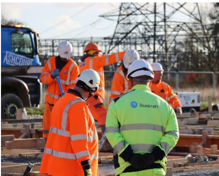
Ashcourt Group have been providing civil construction services and Fenstone have been supplying stone for the project.
